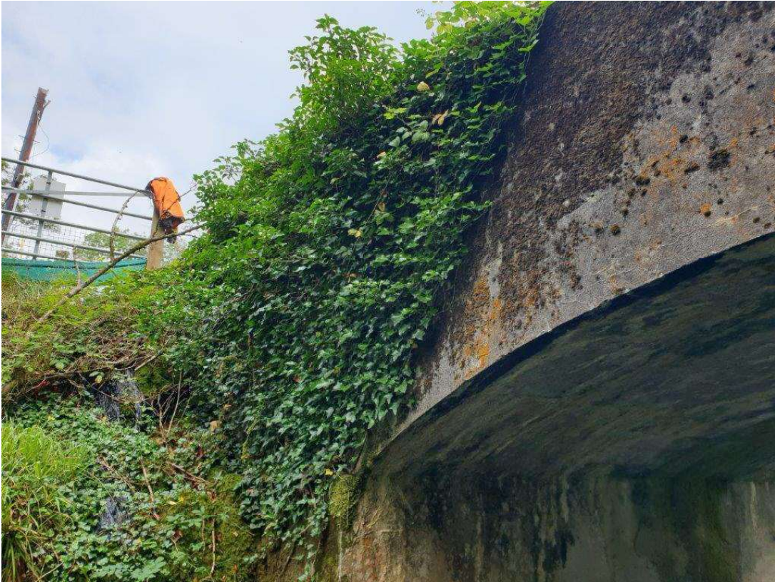
Vegetation growth on the west elevation
