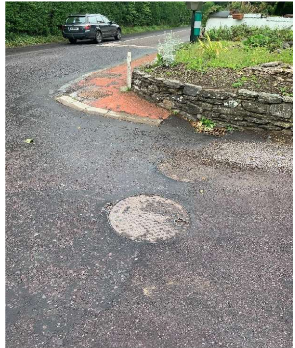
Image : 38 Visible services in the village of Ballvourney
