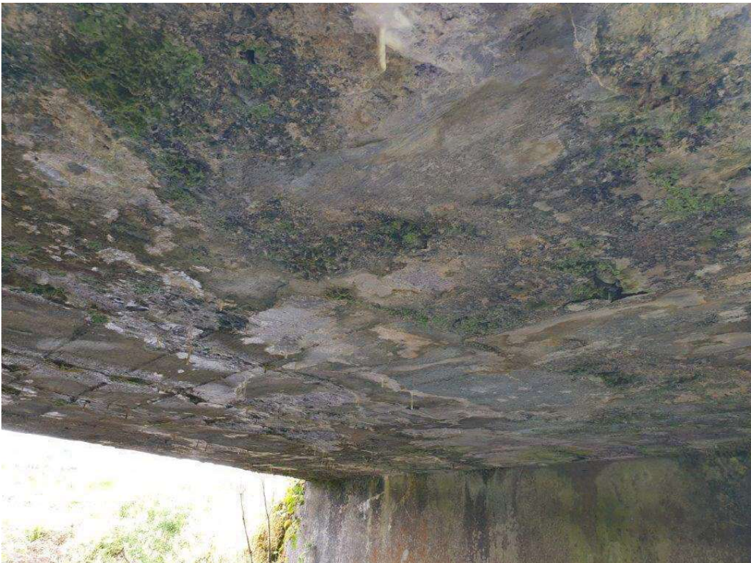
General view of the soffit of the bridge deck showing typical condition
