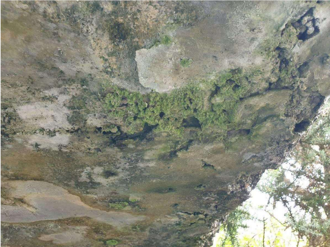
Local scaling of the soffit of the bridge deck
