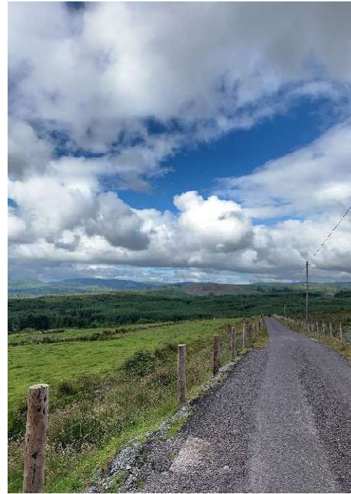
Image : 28 Joint bay on the road here with a links box and communications chambers visible.
