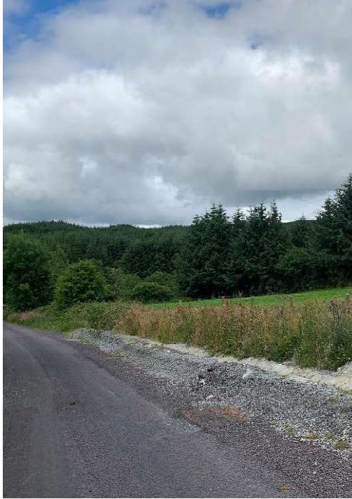
Image : 31 Joint bay on the road here with a links box and communications chambers visible
