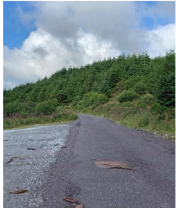
Image : 12 Joint bay on the road here with a links box and communications chambers visible.
