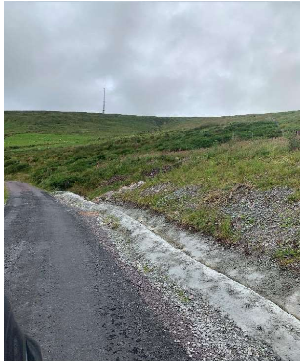
Image : 18 Joint bay on the road here with a links box and communications chambers visible.
