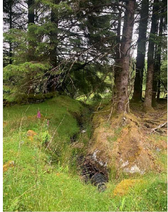
Image : 77 Twin wall UPVC storm pipe crossing under road
