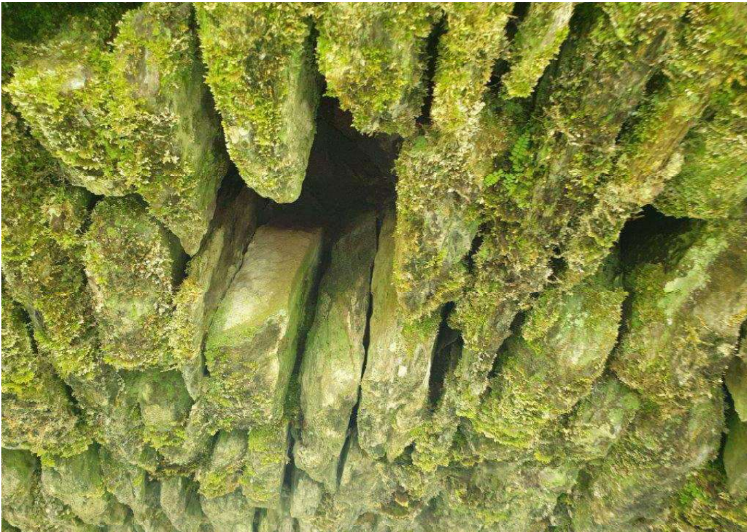
Dropped / missing stones in the arch barrel towards the north face of the bridge
