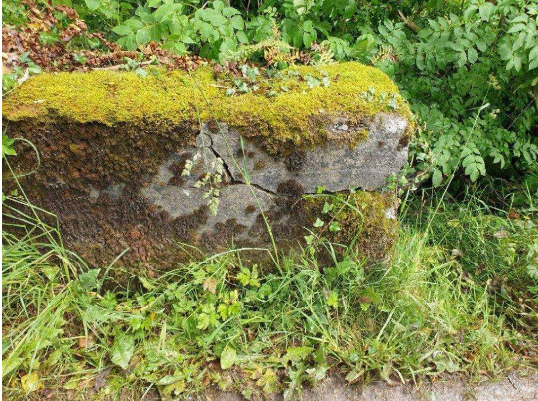
Local damage to the west parapet
