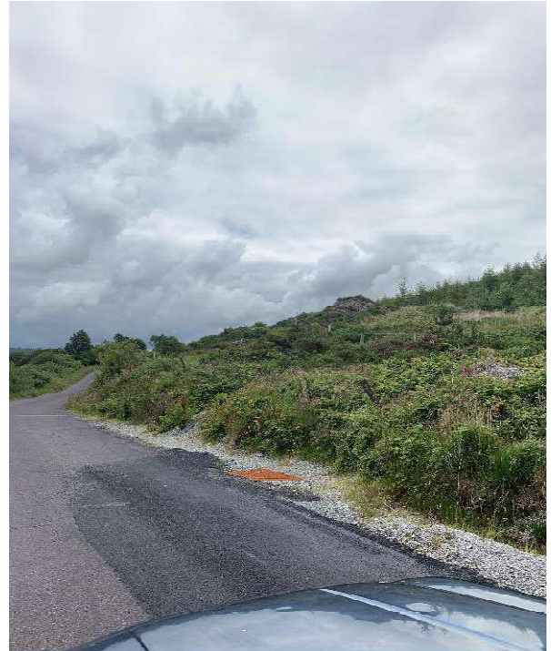
Image : 52 Joint bay on the RHS of the road at this location with a links box and communications chambers visible.
