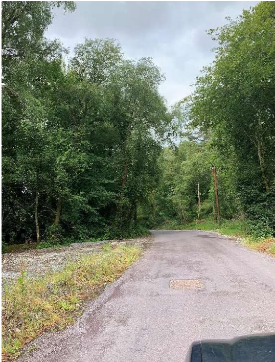
Image : 37 Joint bay on the road here with a links box and communications chambers visible.
