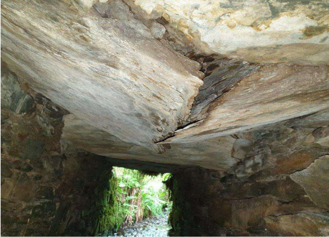
Soffit of bridge deck - viewed from D/S. Collapsed Flagstone (north span)
