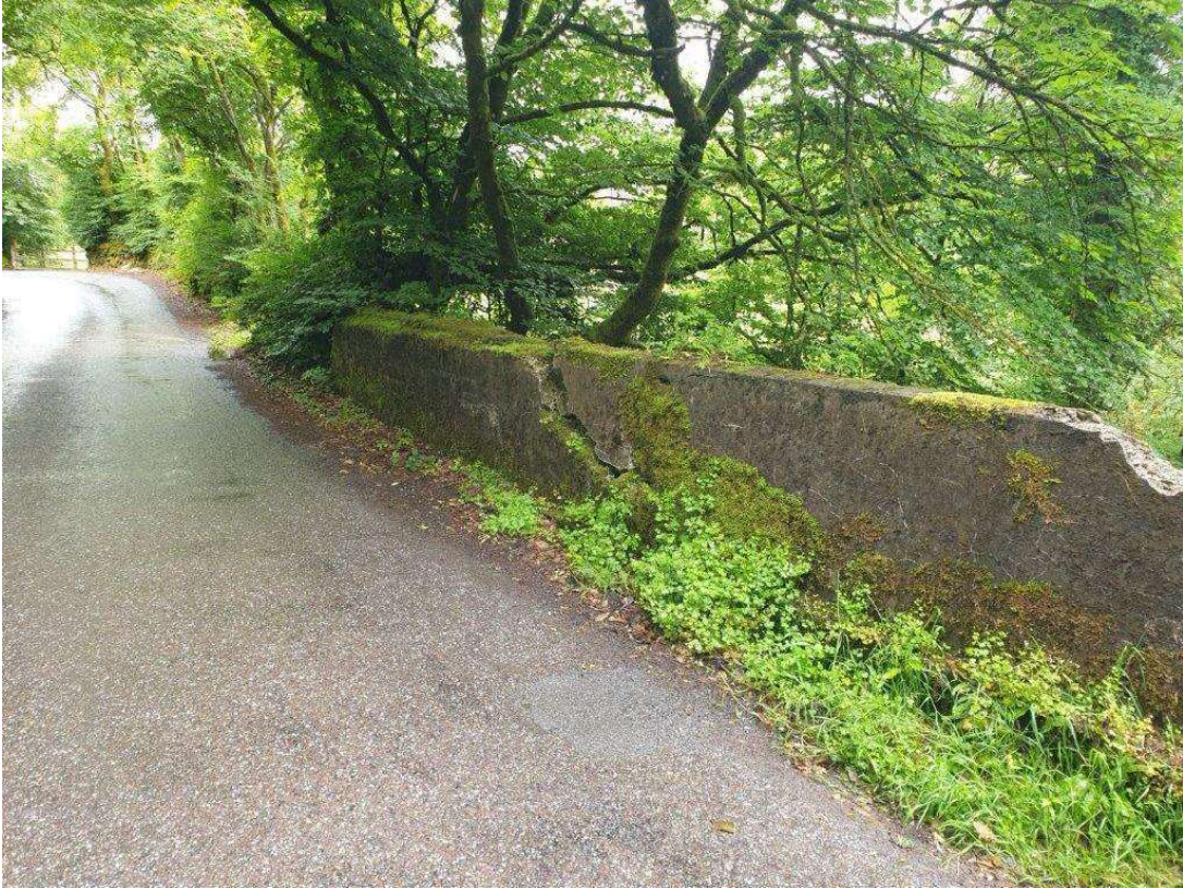
South parapet showing partial collapse extending from the centre of the bridge
