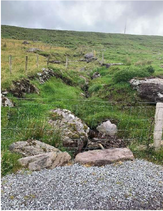
Image : 21 Storm water pipe crossing under road at this location
