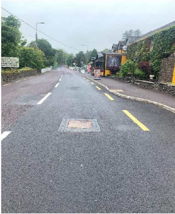
Image : 39 Visible services in the village of Ballvourney
