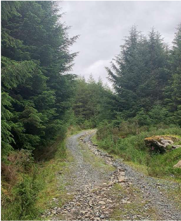
Image : 72 Forestry track on Coillte lands very steep and heavily rutted
