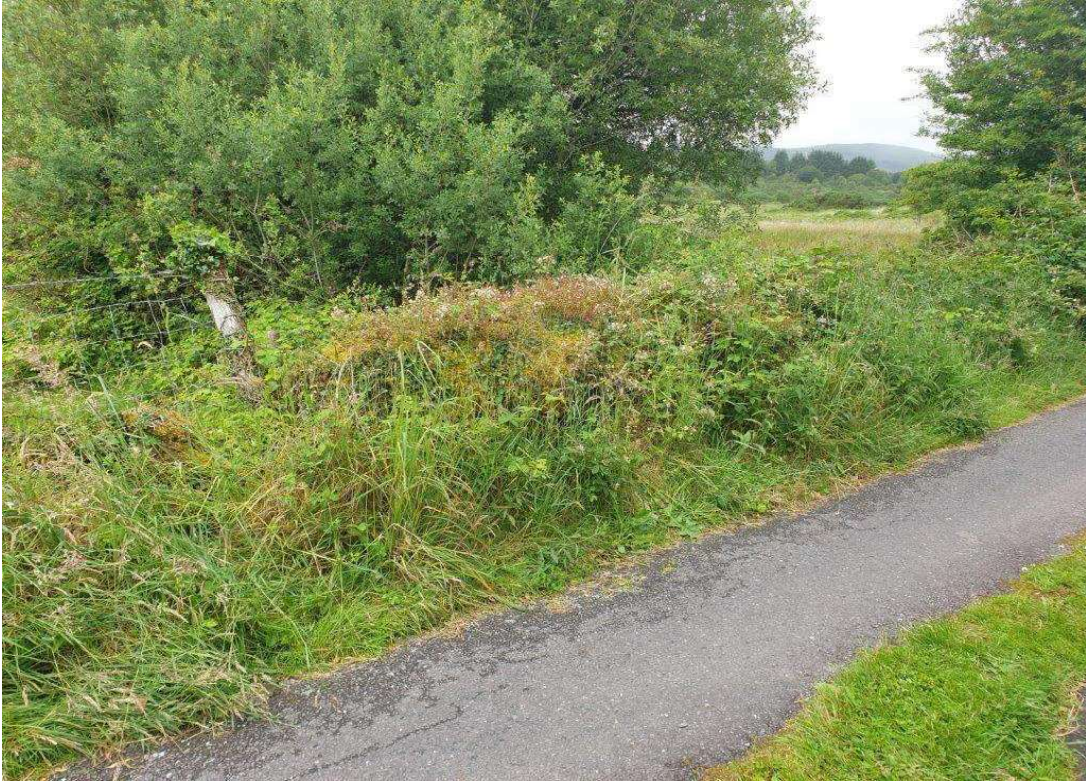
Stone masonry wall on the D/S side of the bridge in poor condition and very overgrown with vegetation. Masonry block wall on the U/S side of the bridge as seen in previous image,
