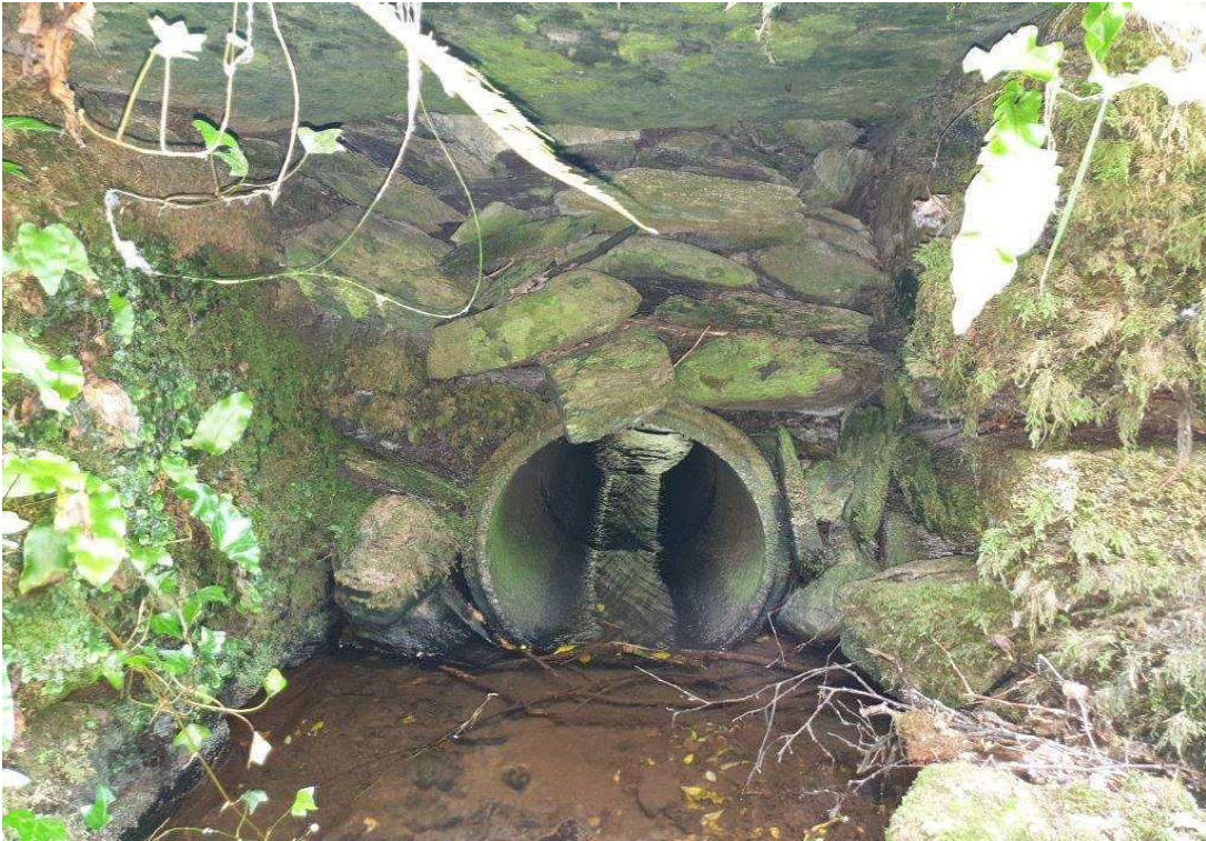
Repair to existing culvert with a 450mm concrete drainage pipe (south span).
