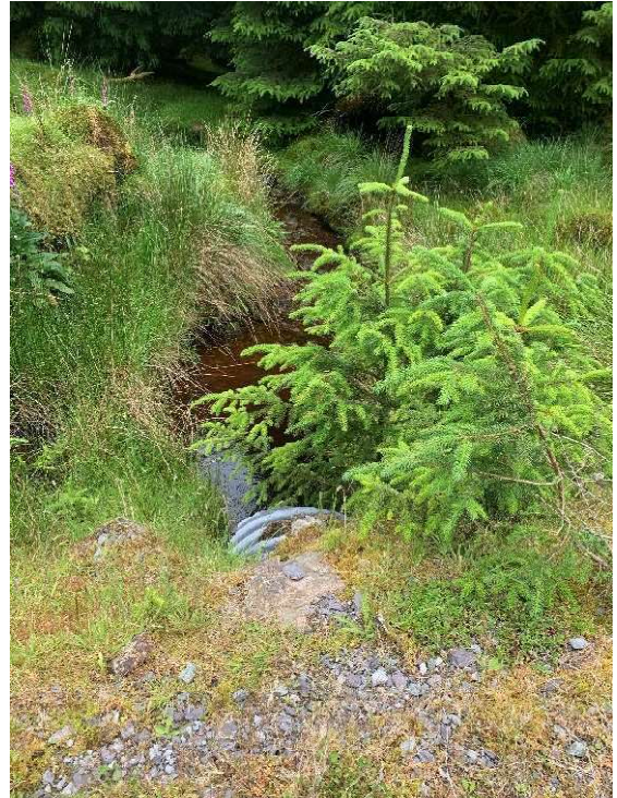
Image : 81 Twin wall UPVC storm pipe crossing under road
